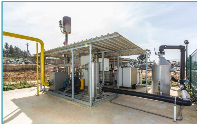
Biogas cleaning unit
