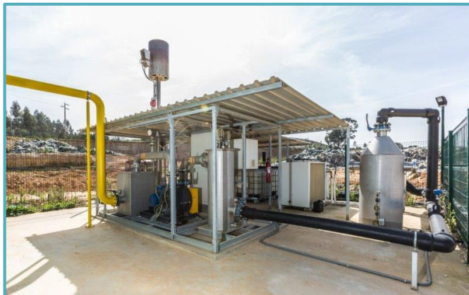
Biogas cleaning unit
